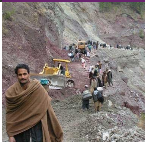
Image above: Neelum Valley Road in Pakistan after the 2005 Kashmir Earthquake (Photo: Professor Dave Petley).
