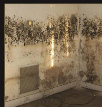
Mould on damp living room wall (Author: Infrogmation)
